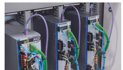
EtherCAT control system
